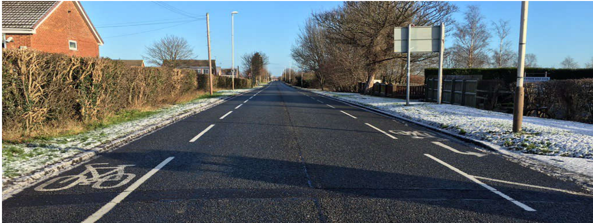
Figure 10 – Example of road with no centre line
